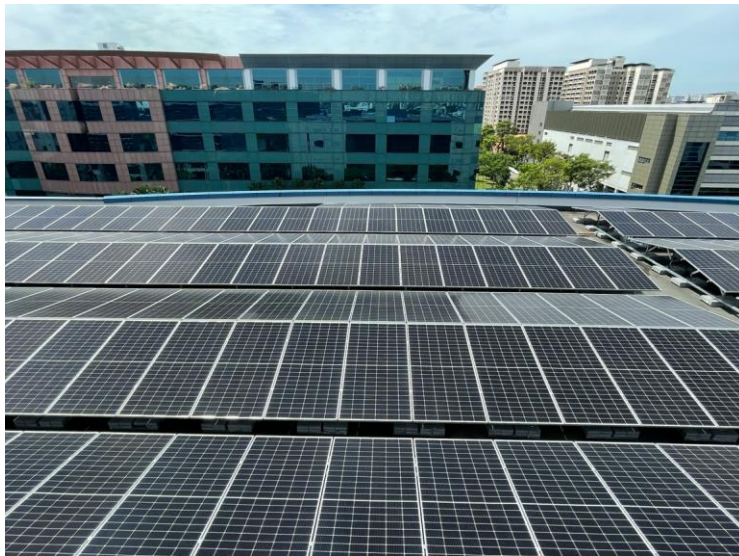
Caption: UTAC's rooftop installation will generate over one million kWh of green energy annually
